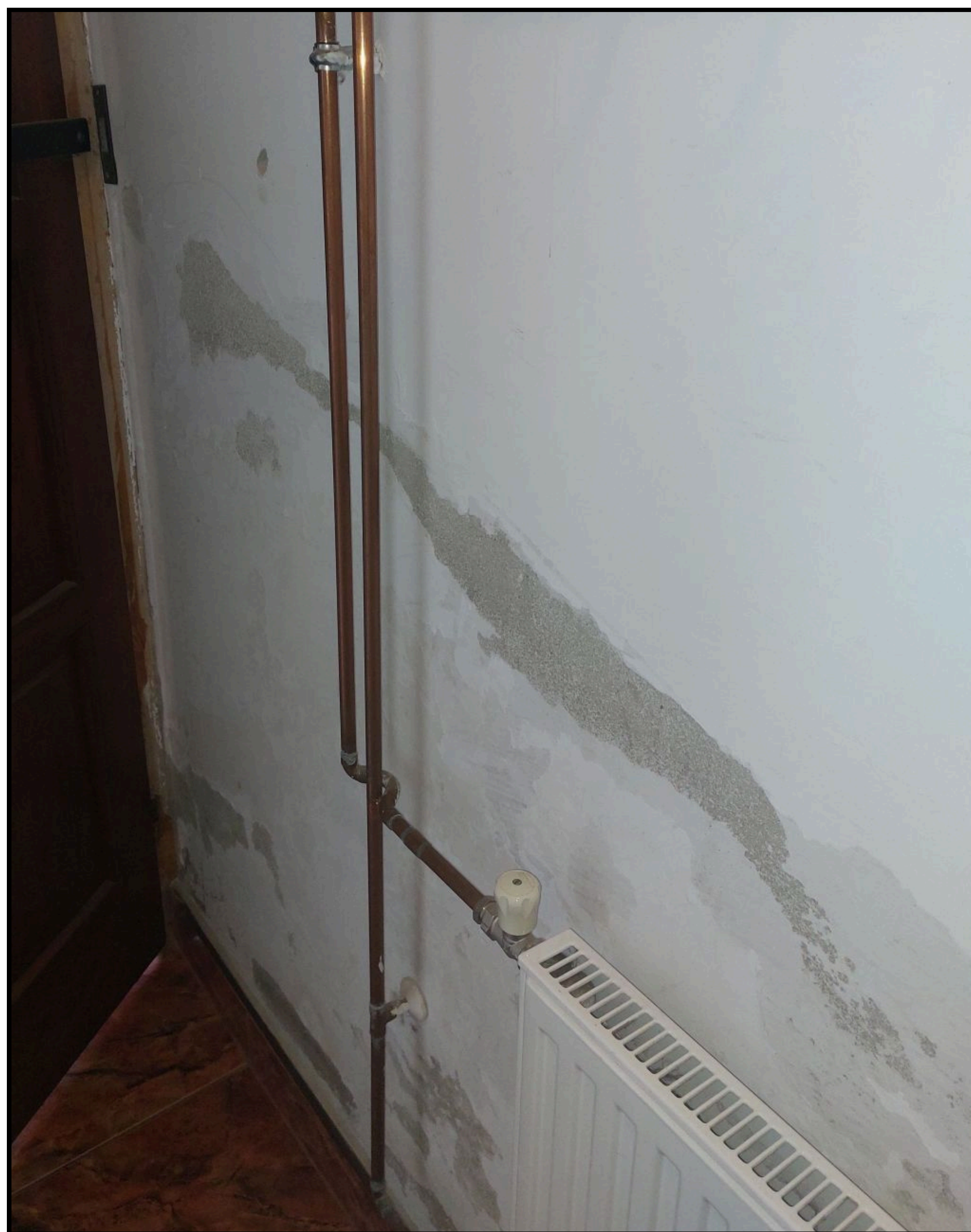
Picture 2: The original water-damaged wall
